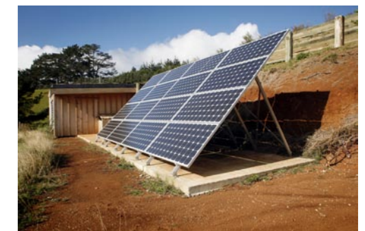
Ten 175-watt photovoltaic panels charge a 48-volt battery bank through an inverter system, which converts the power to 220 volts for the house
